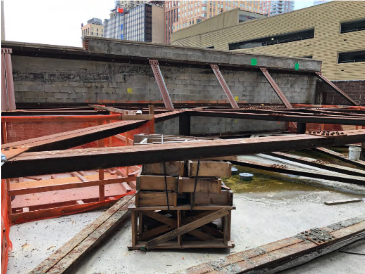
The roof parapet for the southern wall of the Robert and Anne Dickey House. Photo by Michael Young
